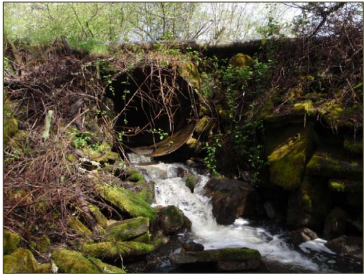
Stream crossing in poor condition on upper Green Valley Creek. This crossing is a barrier to coho salmon passage. Photo courtesy of John Green.
