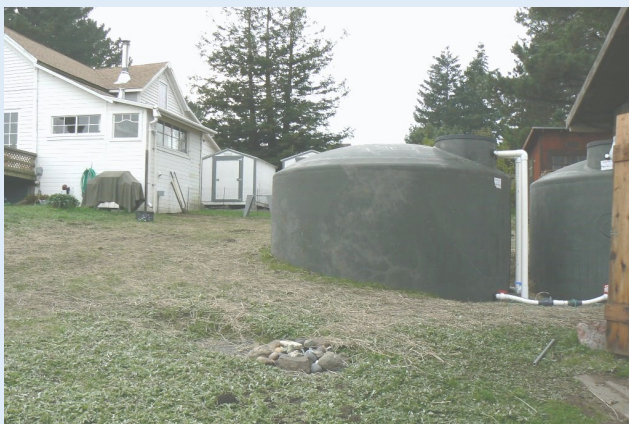
Completed rainwater system, with 5,000-gallon water storage tanks at right and water conveyance downspout and first flush diverter on the house at left.
