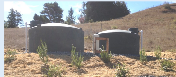
5,000-gallon tanks storing rainwater for dry season irrigation in Bodega.
