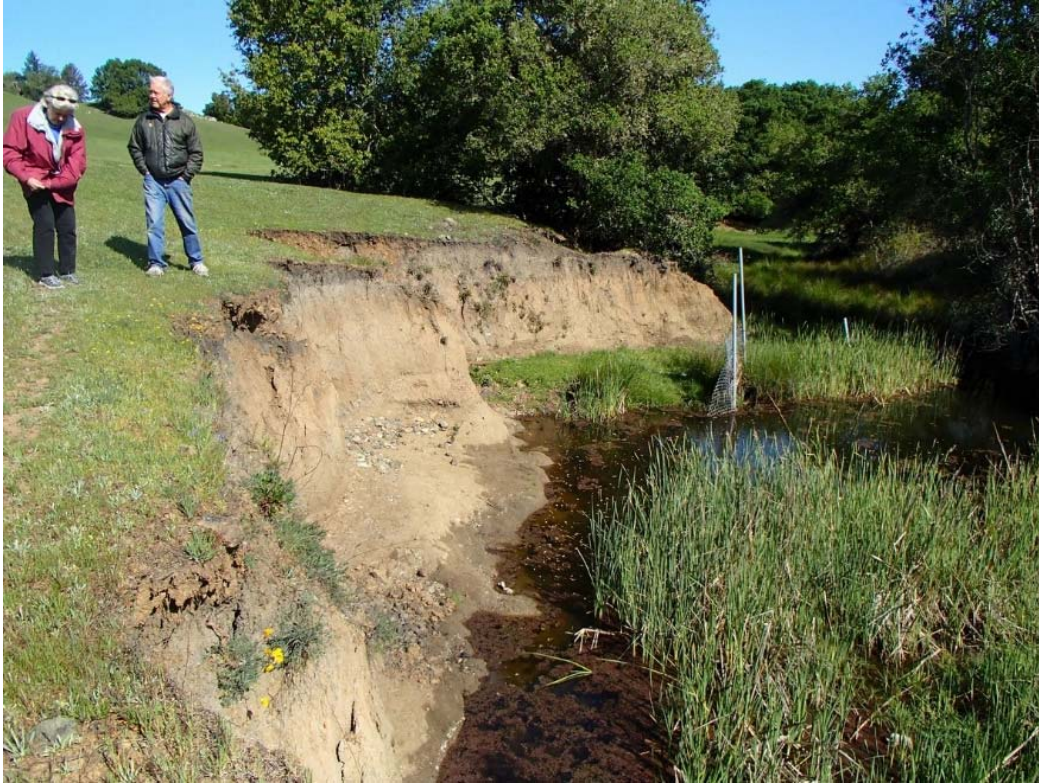
Photo 1. View looking upstream at Site A bank erosion (March 2015).
