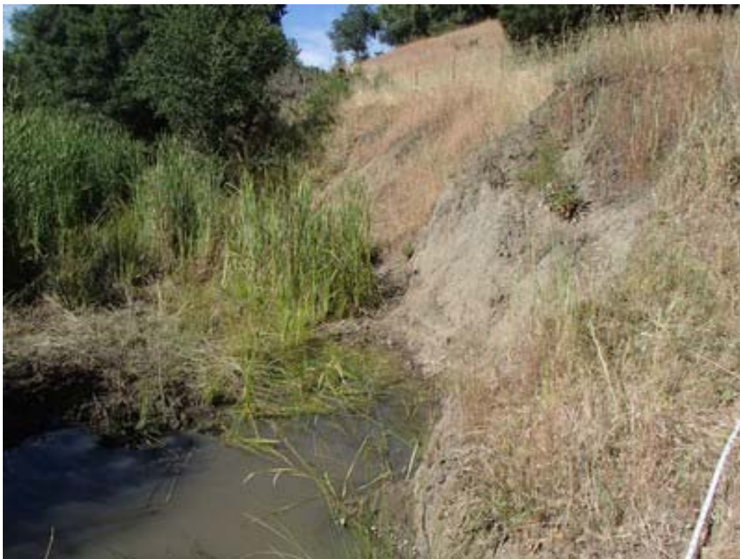
Photo 4. View looking upstream at Site B bank erosion (June 2016)
