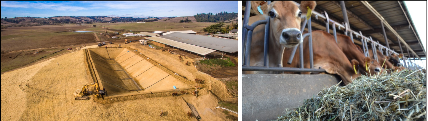
Left: The Hughes Dairy's 1.4 mil gal water storage tank will be constructed by December 2015. Right: The Hughes' Jersey dairy cows who will be drinking the captured rainwater in the summer of 2016.
